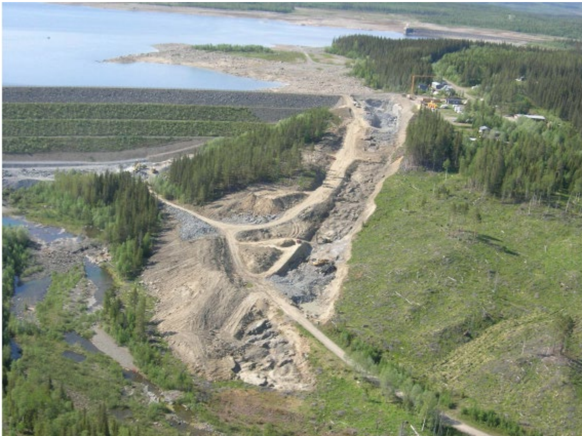
Figure 7. Ongoing construction work to provide the Håckren dam with a new surface spillway. (Photo: Vattenregleringsföretagen, 2006)
